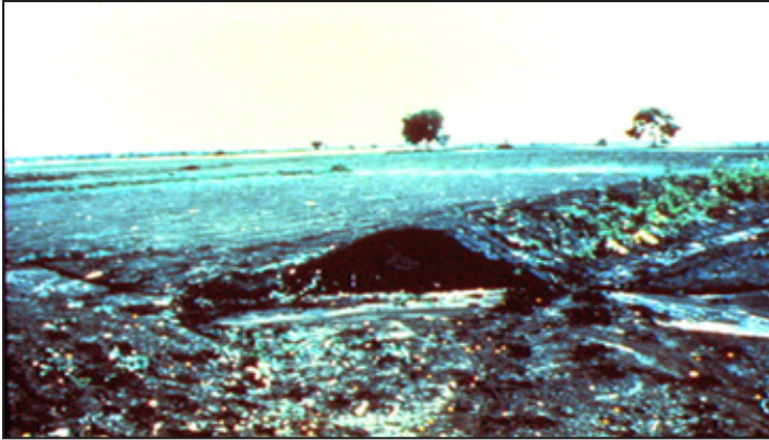
Photo 9a Not only has the constructed bank failed, but the cotton crop that the bank was constructed to protect has also failed. Before this bank's failure, the constructed system trapped too much water, flooding the entire area. Because cotton cannot tolerate poor drainage, the crop failed completely.
