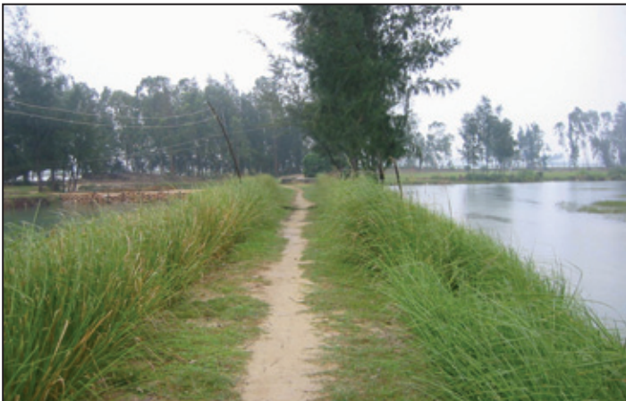
Photo 36. Vetiver hedgerows used to protect both sides of a canal bank in Vietnam. (Tran Tan Van).
