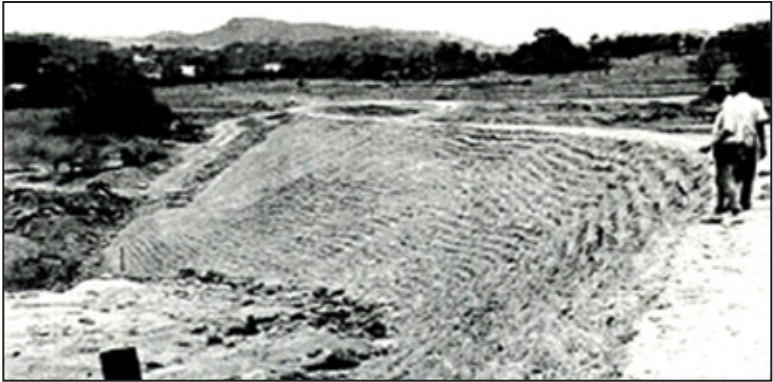
Photo 38b. Vetiver grass planted on this dam wall protects the down slope from erosion.
