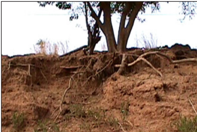
Photo 2. Loss of soil exposes roots.
