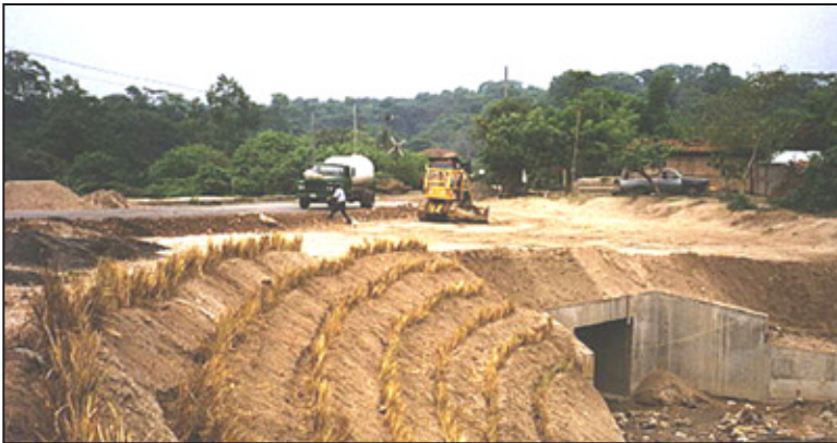
Photo 35. In El Salvador, newly planted vetiver hedgerows protect the approaches to a small bridge.
